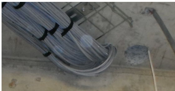
a) left-hand hole full of cables (c.f. 'percentage fill' limits)
