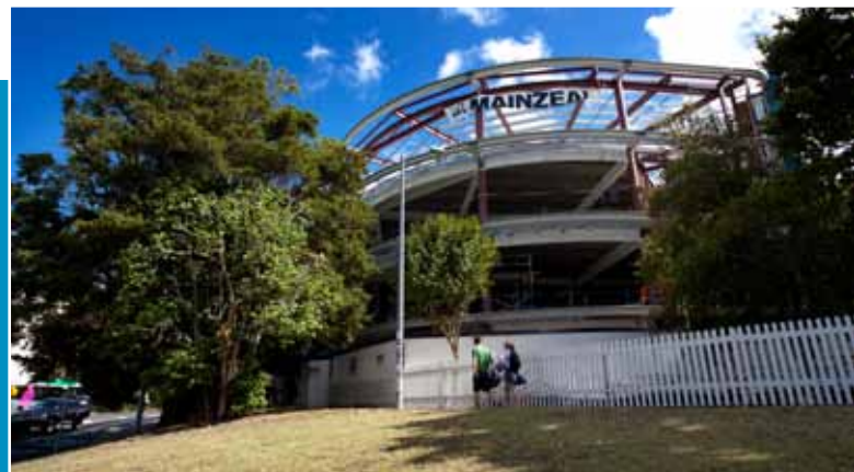
The extension to the School of Biological Sciences will be completed late in 2010.
